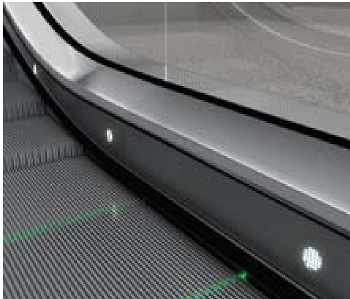
Photograph 4 — Brush deflector between step and skirt
