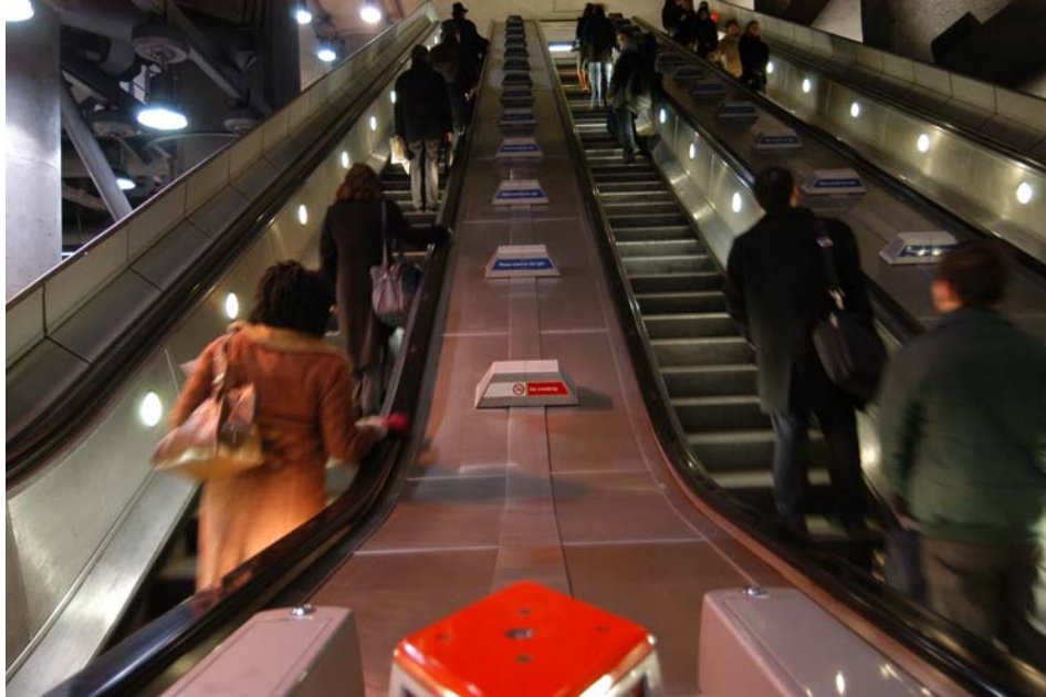
Photograph 1 — Escalator (Courtesy London Underground)
